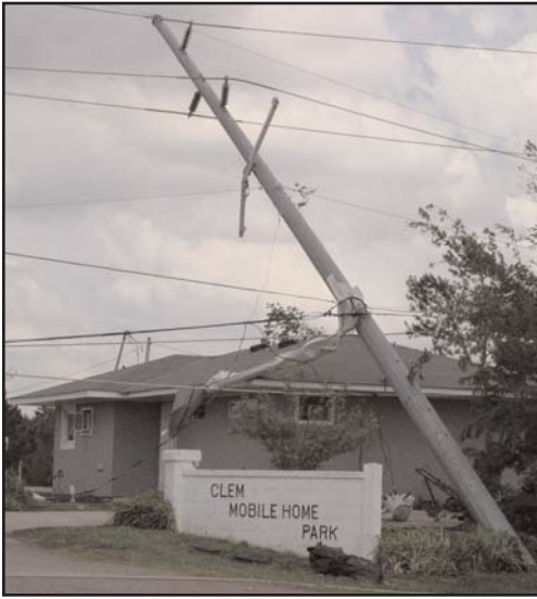
Power lines destroyed in the City of Athens
